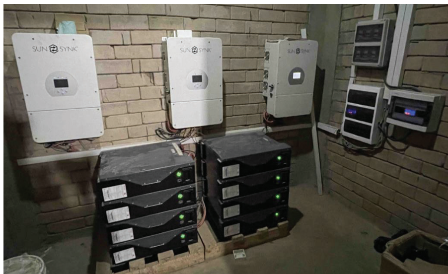
Fig. 13. A state-of-the-art Mbaata solar mini-grid control room consists of 3 SunSynk inverters (3-phase AC) and WECS lithium-based batteries. (Credit: Robert Foster)
