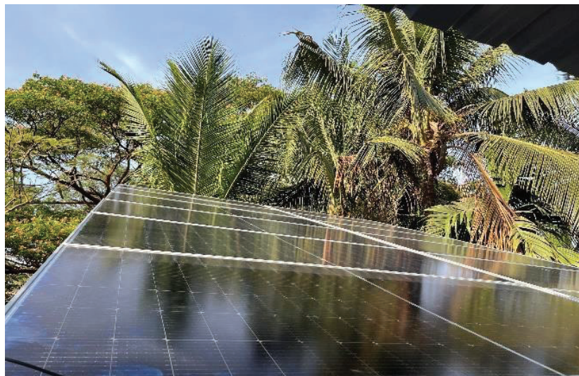
Fig 4. (a) Solar PV system design. (b) Installed bifacial solar panels. (Credit: Dany Hemanth)
