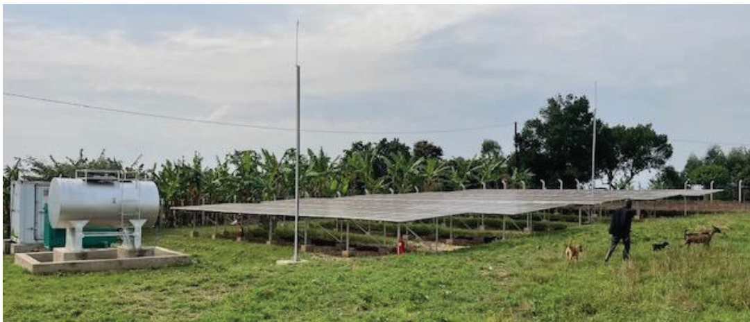
Fig. 15. The Katarwe village 56-kWp solar mini-grid was installed by NRECA in 2022 for USAID Power Africa and operated by the local KRECS utility. This system provides 3-phase power to 176 households, several small stores, two dairies, a coffee factory, and a telcom mast. (Credit: Robert Foster)
