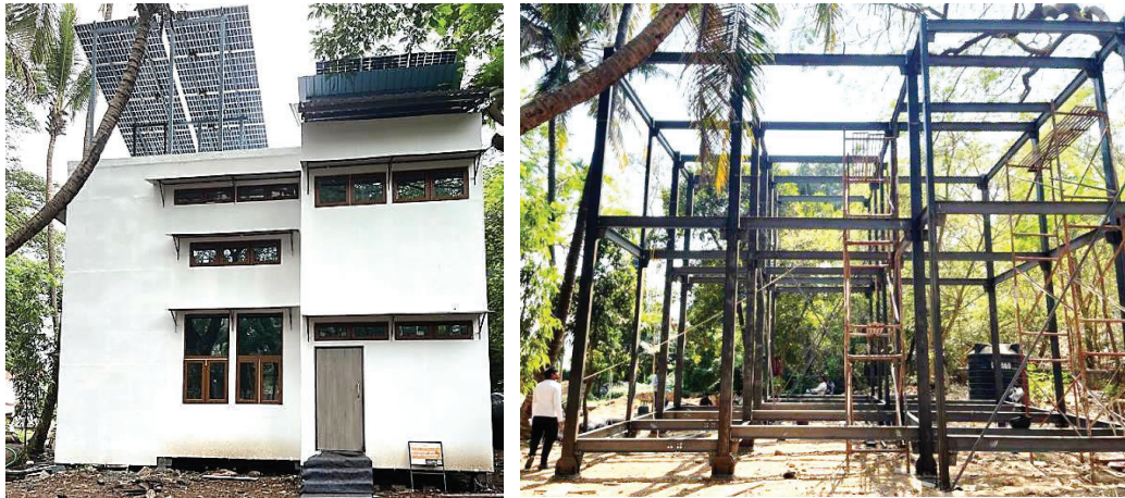
Fig 1. (a) Exterior view after completion. (b) Steel structure of Project Vivaan. (Credit: Prabhat Sharma)
