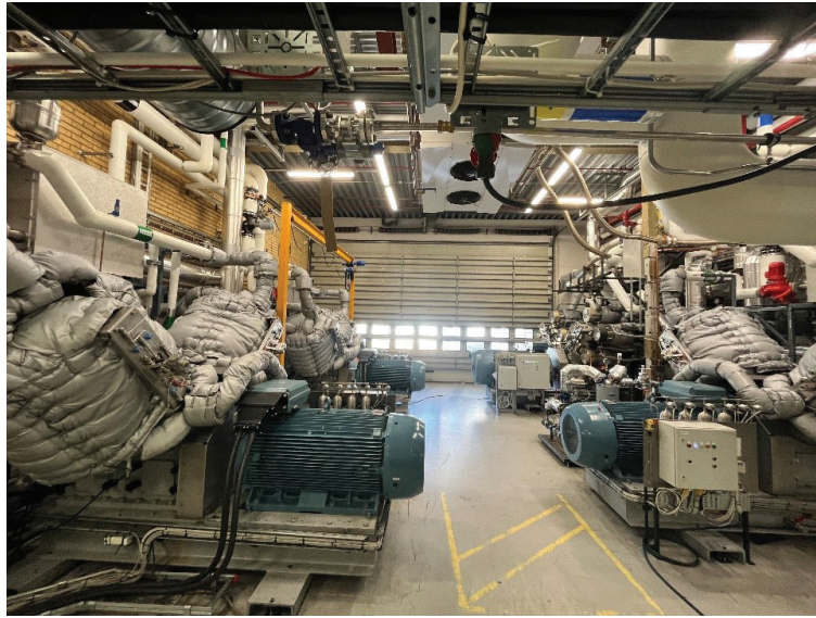
Figure 1: Four HighLift high-temperature heat pumps at AstraZeneca’s R&D center, Gothenburg, Sweden.
