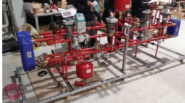
Figure A.2: Bidirectional substation prototype object of the experimental campaign
