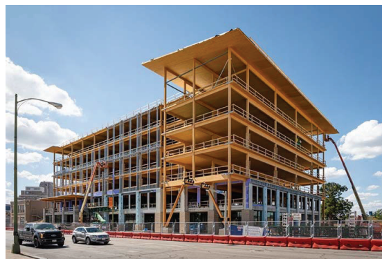
Figure 2: The Soto Building, San Antonio, Texas; Architect: Lake|Flato and BOKA Powell; Engineer: StructureCraft
