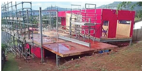
Figure 3: Construction of a CLT residential project in Cairns, depicting the steel framing and ground floor CLT panels with scaffolding and the weather resistant membrane visible
