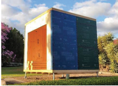
Figure 5: The CLT micro-unit during the ‘construction’ period. The location of the sensor arrays on the interior CLT surface, the 2 WRB types, as well as the exposed CLT surfaces, edge grains, and rough door opening are visible
