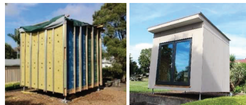
Figure 1: The CLT micro-unit's shown before cladding is installed (left) and after installation (right)
