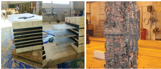
Figure 11: Sealed slots and gaps using intumescent fire strips.
