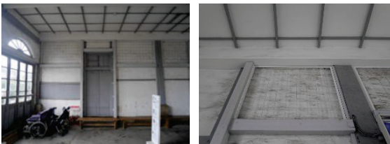
Figure 10: Reinforcements at the East Cocoon Warehouse (left: zoom out view, right: zoom in view), (Date of shooting: July 4, 2022)
