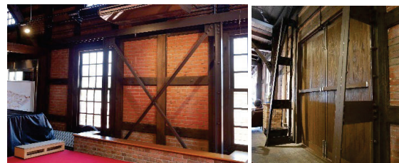
Figure 7: Reinforcements of the Former Kabuto Beer Factory (left: steel frame and brace, right: steel buttresses)
