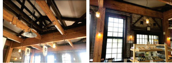
Figure 11: Reinforcements at the Former Engine Room of Kosaka Mine Manufacturing Division: interior view (Date of shooting: Sep. 10, 2019)
