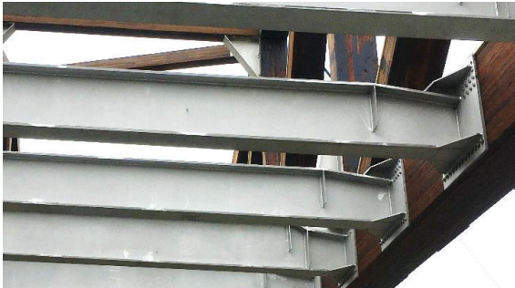
Figure 12: Floor beams connected to lower chord. Photo: Viggo Jakobsen, Consto Nord AS
