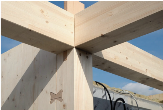
Figure 11: Construction detail, Collegium Academicum. DGJ Architektur, and photograph: Hans Drexler, DGJ Architektur, 2018.
