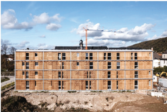
Figure 10: Case Study 1: Collegium Academicum in Heidelberg, Germany, designed by DGJ Architektur, Photographs: Copyright Thilo Ross Urh. Nr. 4026999.
