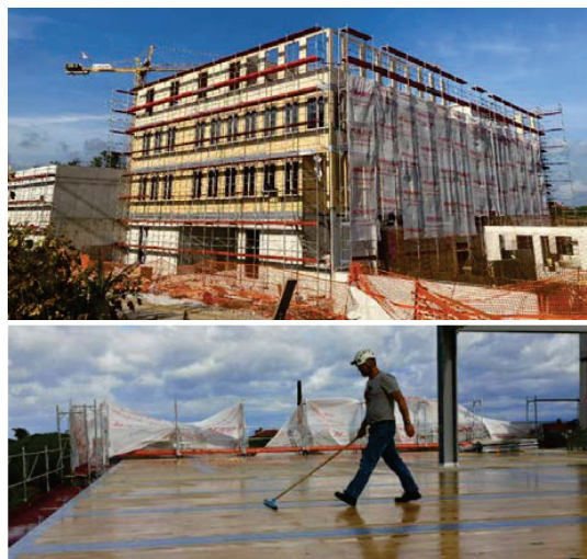
Figure 2: InnoRenew CoE's building, Izola, Slovenia, during construction (up), detail of the CLT floors (bottom)
