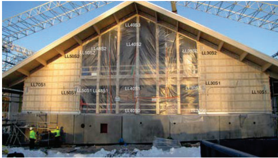
Figure 3: The main building of Hyytiälä Forestry Field Station after removal of construction shelter. Six groups of MC sensors are indicated with black text.
