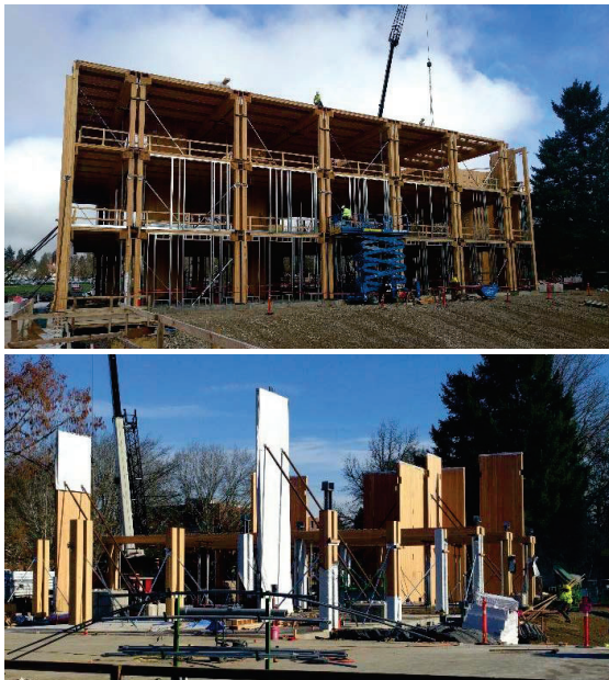
Figure 1: Zone 1 of the PFSC, Corvallis, Oregon, during construction (up), detail of temporary moisture protection during transportation and erection (bottom)
