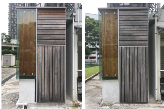
Figure 13 Examples of overall timber cladding discolouration after 28 months exposure (April 2021). Left: N side, Right: S side. The S-side facade exhibits mostly darker colours, while the N-side facade exhibits more moderate and uneven colour changes.
