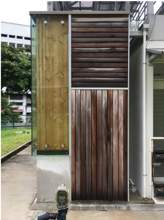
Figure 9: An example of cladding at the SW corner (facing S) a few hours after heavy monsoon driving rain (Nov. 2019). The H-aligned cladding was mostly still wet, while the V-aligned cladding dehydrated relatively quickly.
