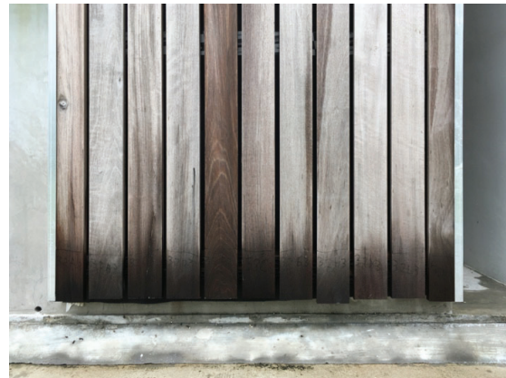
Figure 11: An example of a wet timber cladding base several hours after heavy monsoon driving rainfall (November 2019) – generally, the bottom of the S and W façades became wet and grew darker because of the splash water up to 400 mm above ground level.
