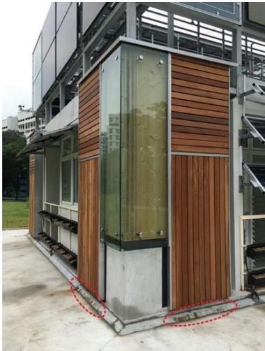
Figure 5: Brown stains on the concrete foundation were observed during the first few months after the installation. They were likely deposited by leached extractives from the red balau timber (red dotted circle, October 2018)
