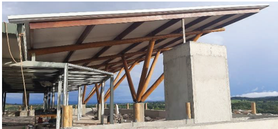
Figure 24: External view of the pole frame
