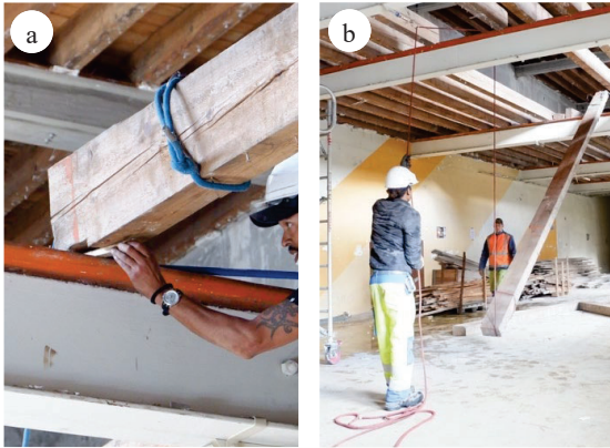
Figure 1.a et 1.b: 1.a shows joists 'denotching' from the I-steel beam. 1.b shows the descending of a joist with the rope system.
