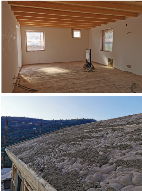
Figure 6: Lime mortar casted in the space between floor beams (up) and on the top of the roof (below)
