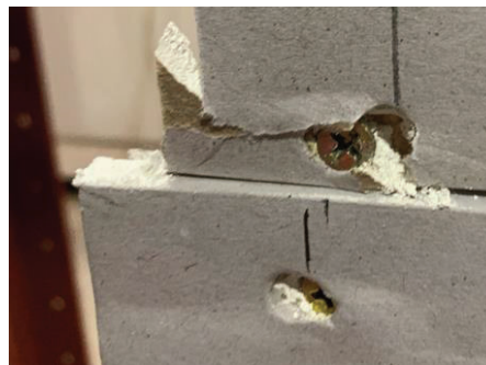
Figure 7: Plasterboard Damage, Test Panel P2.1.
