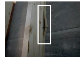
Figure 26: Cracks in the furring strips
