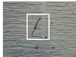
Figure 25: Cracks from around nails
