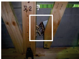
Figure 30: Fascia plate screws missing
