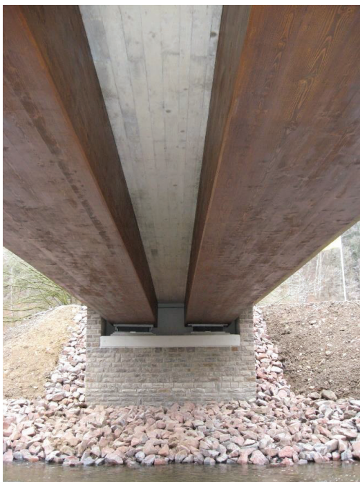
Figure 10: Bottom view of a timber-concrete composite bridge (Birkbergbridge, Germany) showing a sufficient distance between superstructure, support bench and ground for good ventilation and easy inspection (photo: A. Simon)
