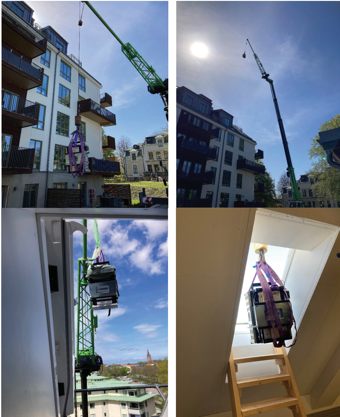
Figure 6. Lift off the 140 kg shaker from the ground to the top floor position through a small attic window.
