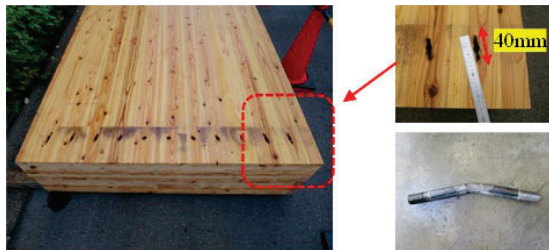
Figure 7: Inside of S-M16 CLT panel (left: back side of CLT panel, top right: bolt track, bottom right: bent bolt)
