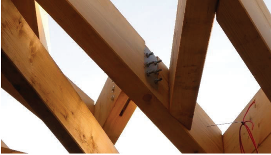
Figure 9: Detail with slotted-in steel plates of Frans Masereel Centrum in Kasterlee, Belgium
