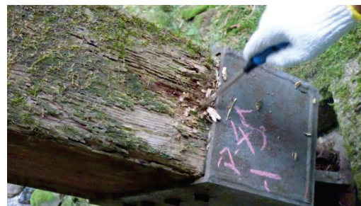
Figure 12: Decay at the end of arch rib
