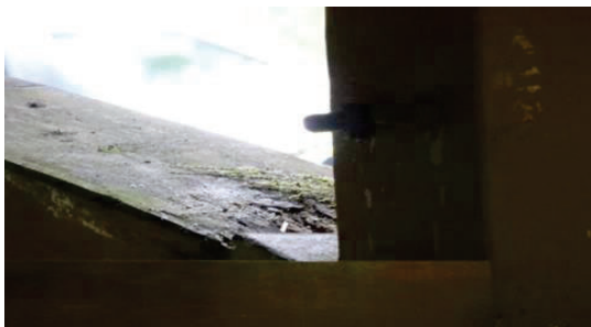
Figure 14: Decay of connection between spandrel column and arch rib
