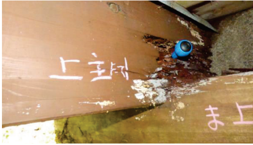
Figure 13: Decay of connection between longitudinal beam and sleeper beam
