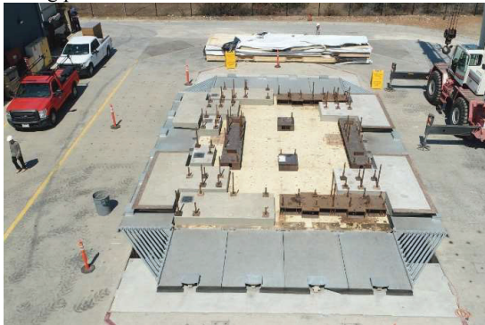
Figure 3: Foundation system added on the NHERI@UCSD outdoor shake table before construction started
