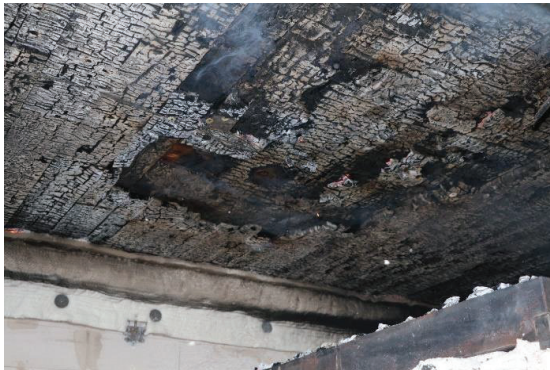
Figure 13: Bond-line failure leading to premature char fall-off in experiment without beam.
