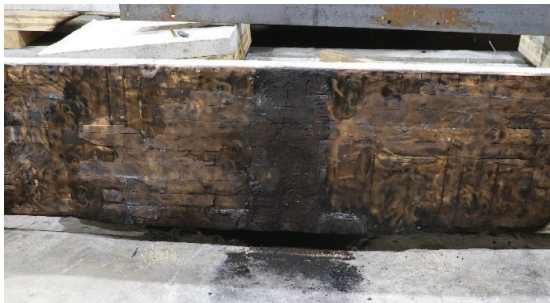
Figure 10: Char layer removed on the entire bottom surface of Slab 1
