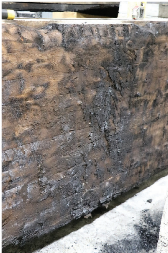
Figure 11: Residual CLT section at the midspan of Slab 2 after removing the char layer
