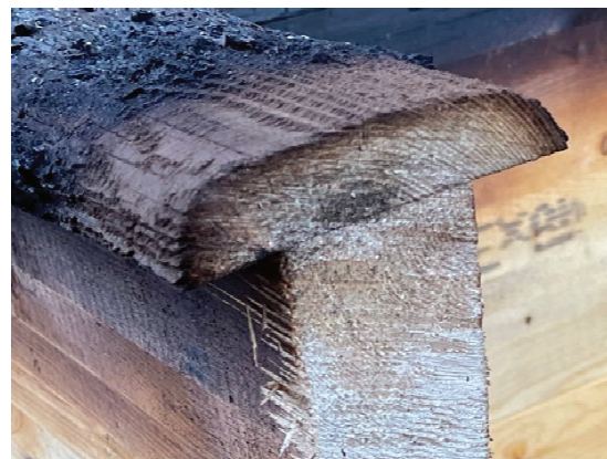
Figure 11: The residual cross-sections of the flanges after the fire experiment. The main load-bearing beam is discoloured but not charred
