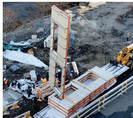
Figure 1: CLT exterior wall assembly prefabricated off-site being lifted at site. CLT forms the support for the thermal and water barriers to the exterior face (image credit: Blomgren)
