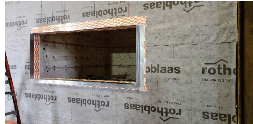
Figure 11: Test 1 set up, showing installation of window frame surround and sealing tape, prior to mineral wool overlay (image credit: Blomgren)
