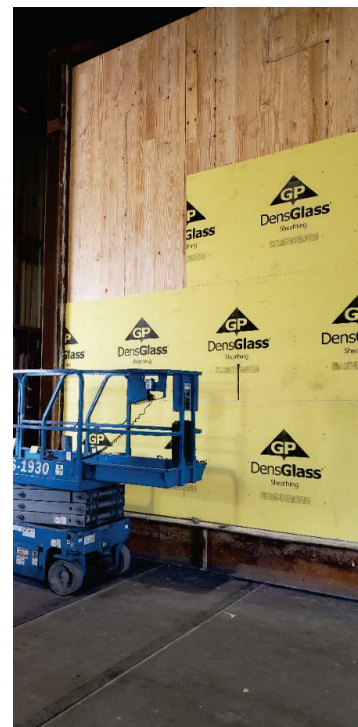
Figure 7: Test 1 set up, showing installation of fire rated gypsum board (image credit: Barber)
