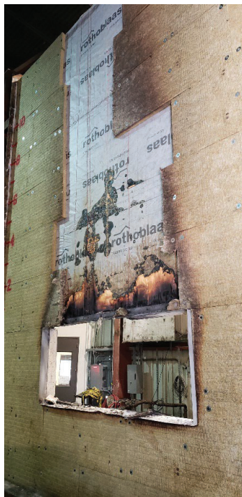
Figure 19: Test 2 completed, showing extent of damage, with mineral wool manually removed. Damage can be compared with that of Test 1, shown in Figure 16 (image credit: Blomgren)
