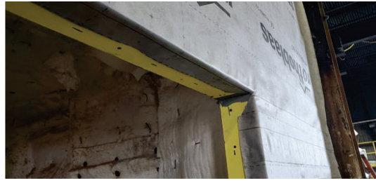
Figure 10: Test 1 set up, close up of gypsum board to window edge and WRB wrap-around (image credit: Barber)
