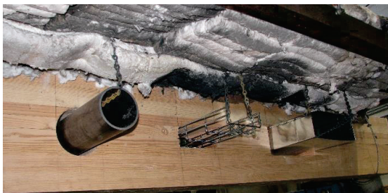
Figure 3: Glulam beam (Type C) with penetrations for a pipe, cable tray and duct (left to right).
