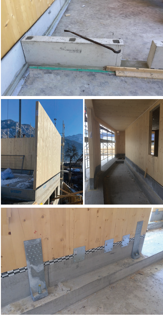
Figure 3: on site construction phases: levelling and anchoring (top picture); placing the CLT walls on the top of the prefabricated beams (central picture); connecting timber wall to the prefabricated system (bottom picture)
