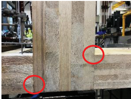
Figure 12: Localised crushing to floor at both walls (specimen with generic bracket B1 UoB at C4)
