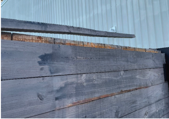
Figure 12: Delamination of top of CLT noise barrier
