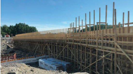
Figure 1: Examples of salvaged wooden materials; cut-offs from a housing company (top) and falsework for a concrete bridge (bottom).
