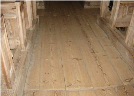
Figure 3: The dimensions of wooden planks of Petäjävesi Old Church floor are large, which was the standard at that time when the sawing was not industrial as today. The surface of the floor has worn unevenly.
