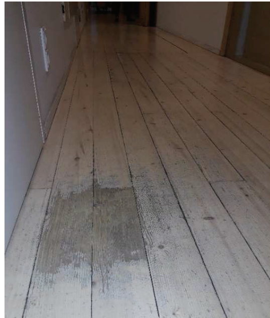
Figure 7: The wearing of the floor in front of a frequently used cabinet, has been intense compared to the surrounded floor.
