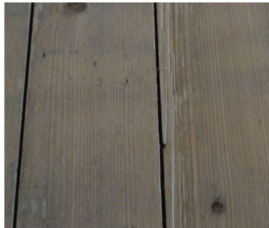
Figure 8: Splitting of the boards in has been a problem in Viikki Church.
