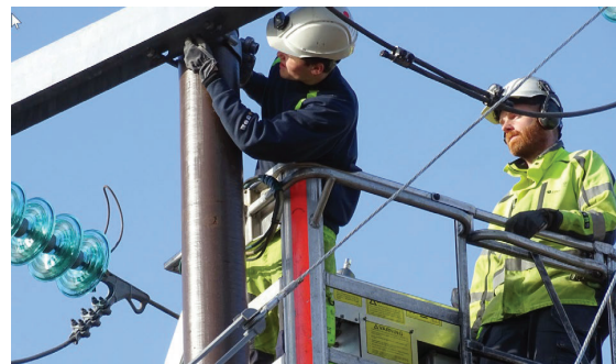
Figure 4: Fitters from Linde Energi using French bolts with mastic to prevent sliding and rotation of cross arm fitting.
