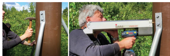
Figure 10: Anomalous sound from hammer was followed up using resistograph, in turn showing normal values.
